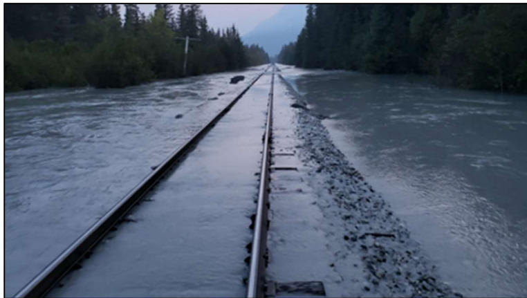
Figure 6: Tracks Submerged during a Flood Event
