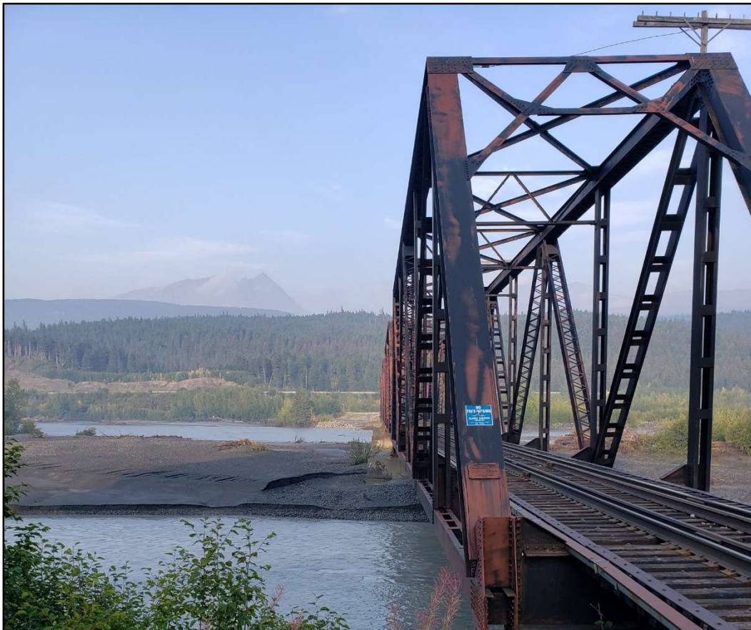
Figure 4: Sediment Upstream of MP 14.5 Bridge
