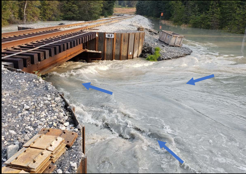
MP 16.2 Bridge During 2019 Flood -ARRC
