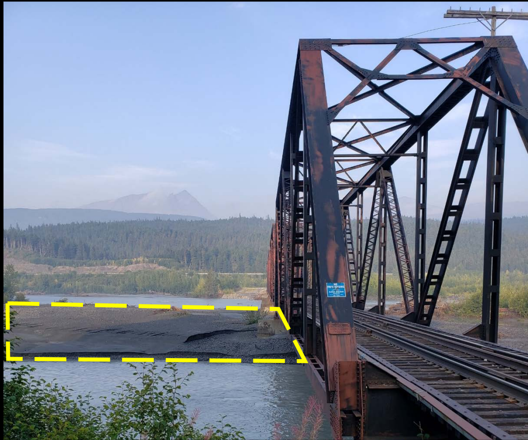
Sediment Upstream of MP 14.5 Bridge
