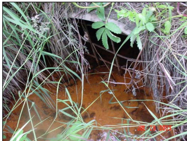
FIGURE 3.2-6 Stagnant Water at Inlet to New Seward Highway Culvert Crossing at Fish Creek (July 2003)
