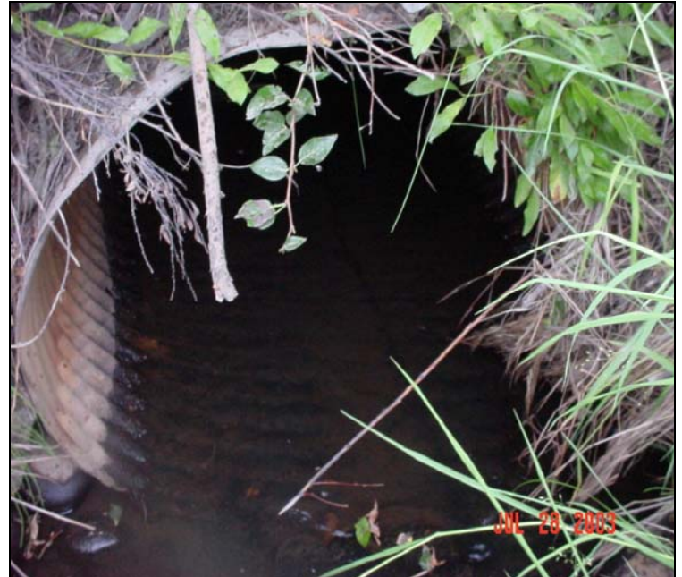
FIGURE 3.2-4 Photograph of Sampling Location on North Fork of Little Campbell Creek (July 2003)
