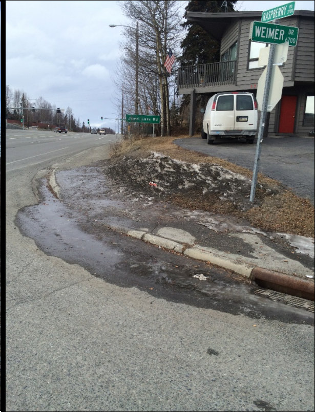
Figure 9: Storm drain along Raspberry Road
