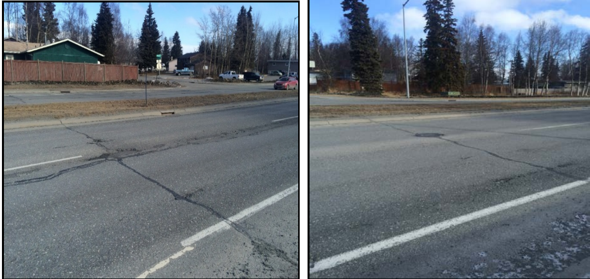
Figures 3 and 4: Distresses in eastbound lanes
