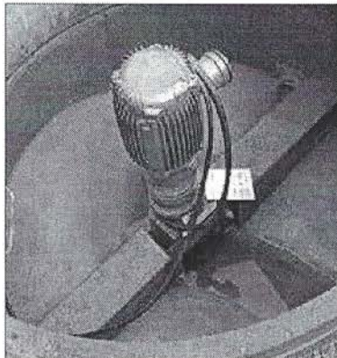
A 3-HYDRO-C Sewage Grinder with Immersible Motor at a Veterinary Clinic
