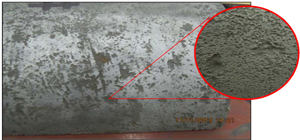
Figure 11 – Condition of Similar Pipe (UAA Corrosion Lab)
