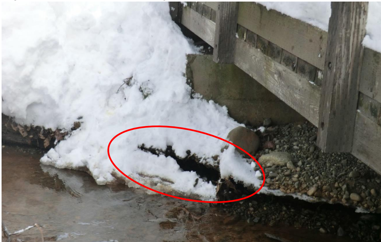
Figure 29. Scour at South Tikishla Bridge
