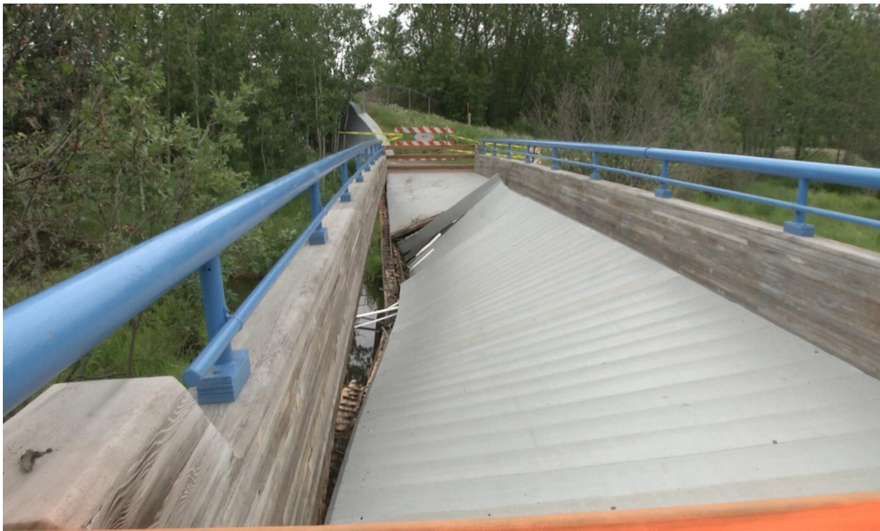
Figure 2. Westchester Lagoon Bridge Failure
