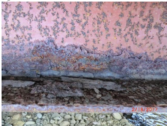
Figure 3: Worst Corrosion on Girders
