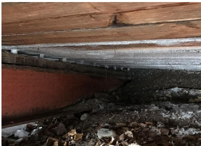
Figure 5. Frame and Girder Separation
