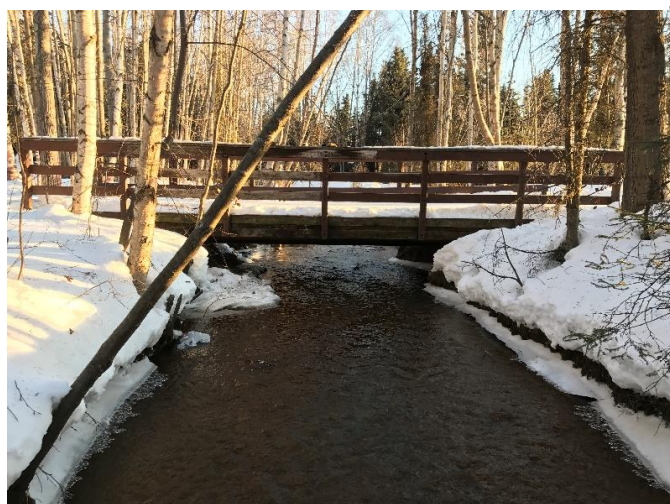
Figure 4: Profile view of Sagging Bridge Frame
